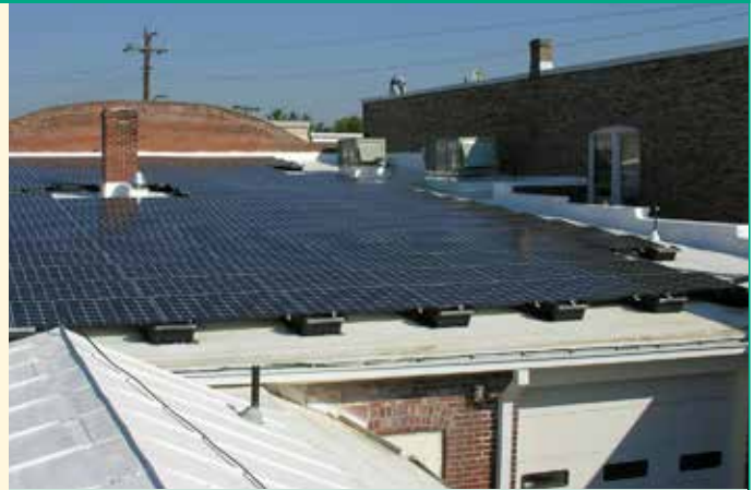
The solar array offsets about 85 percent of the distillery's electrical usage.
